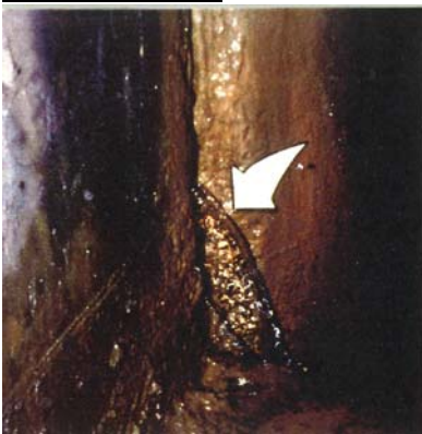
An Example of Water Intrusion
