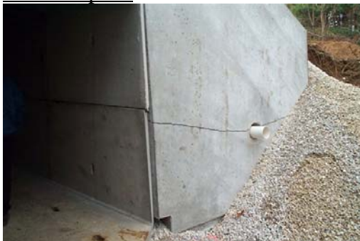
Crack in Concrete Retaining Wall
