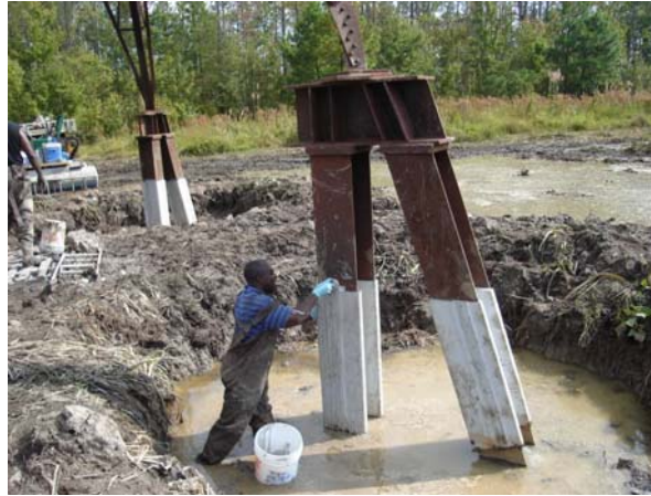
Figure 11: Steel H Piles repaired with an H-shaped fiberglass jacket.
