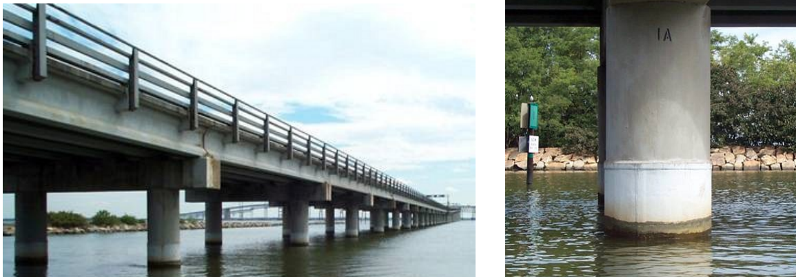
Figure 7: The Chesapeake Bay Bridge, pictured 20 years later. The piles restoration still looks as good as the day it was completed.
