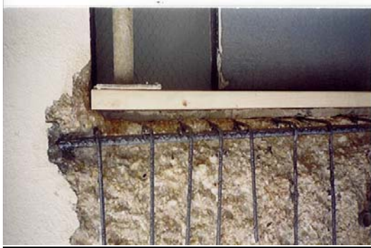
View of a Small Vertical Spall
