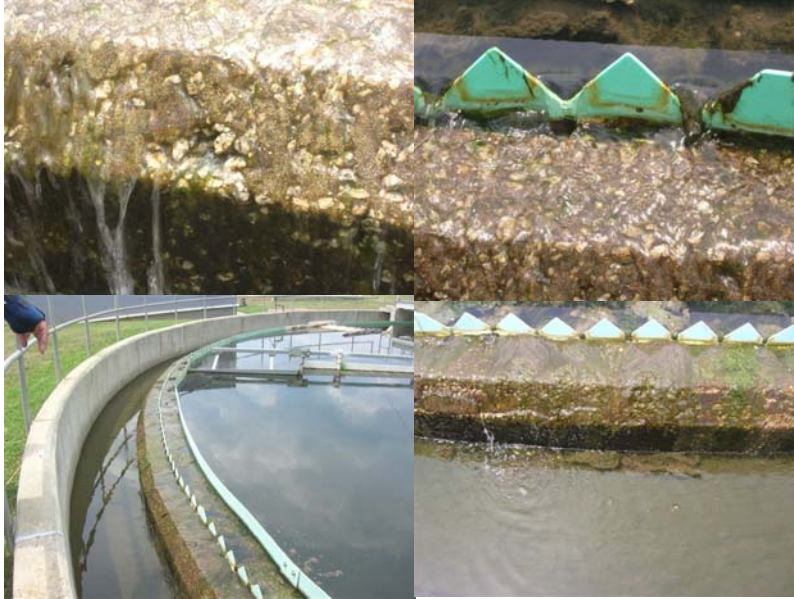
Erosion of Concrete, Resulting in Exposed Aggregate
