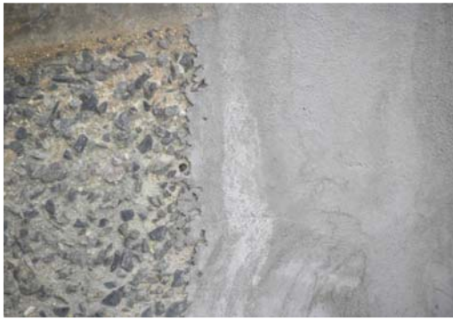
Close-up View of Large Spall
