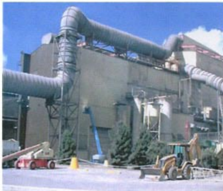
View of melt shop building in the process of being cleaned. High pressure water is used to remove acid cleaner and dirt from cast wall.
