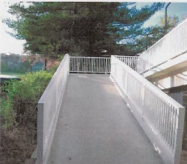
After removal of existing coating and repairs to deck, FX-531 Flexible Epoxy Non-Skid Coating System was applied to the surface.
