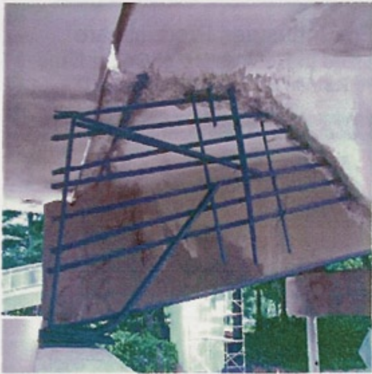
View of deteriorated double tee web after loose concrete has been removed. Strands have been sandblasted and coated with FX-406 Zinc Rich Primer for protection. FX-102 Resilient Fiberfree Bearing Pad was placed on fixed end of double tee and FX-101 Expansion Bearing was placed on opposite end.
