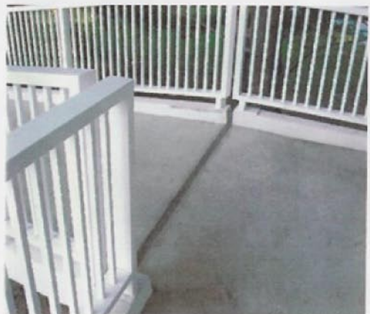
Both sides of joint area were repaired with FX-32 Concrete Mix creating a two inch joint. FX-555 Preformed Sealer was placed in the joint.
