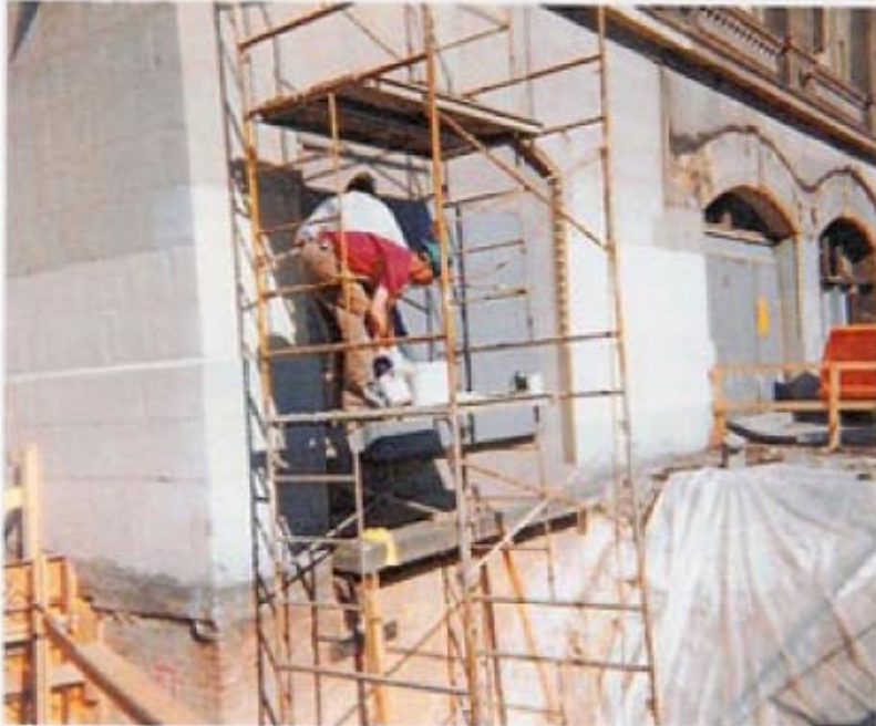
Cracks in the brick foundation wall of the Hippodrome Theater needed to be repaired.
