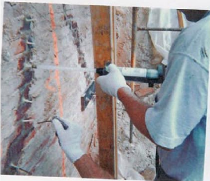
FX-751 LV Epoxy is pumped through ports using air powered handgun and double barrel epoxy tubes with static mixers. (over)
