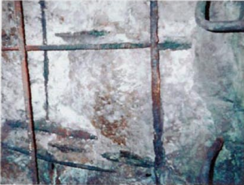
Severely deteriorated concrete ceilings and walls in steam vaults located beneath busy city streets.
