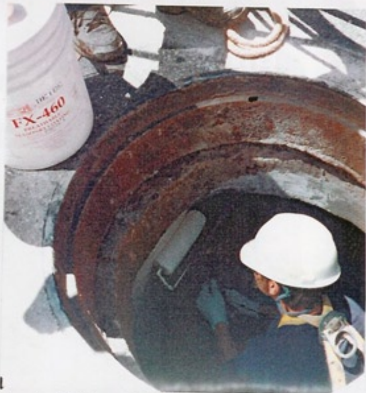
After all patching work has been completed FX-460 Breathable Coating is applied to walls and ceiling of vaults.
