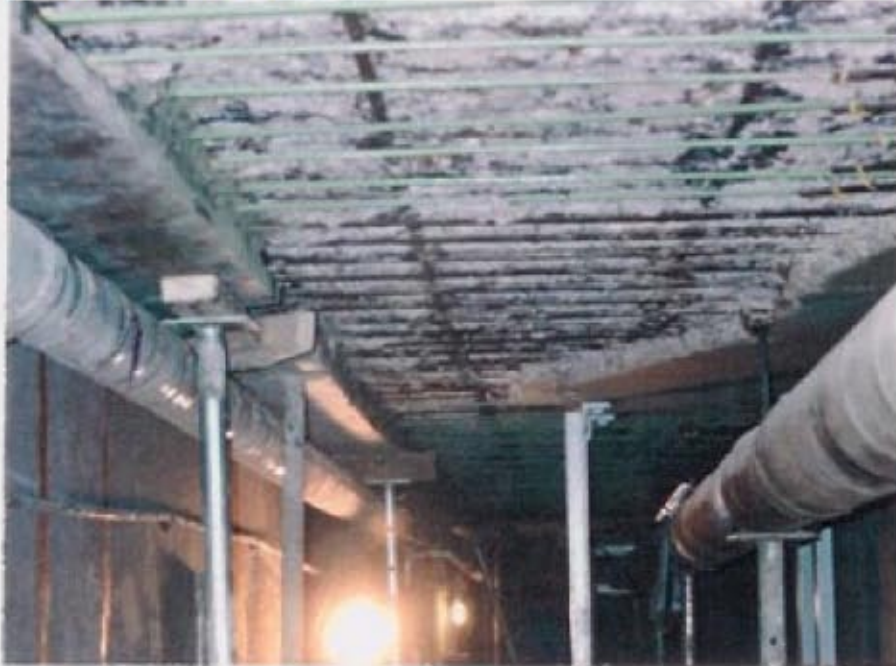
Deteriorated concrete is chipped and removed. New reinforcing steel is placed where necessary.
