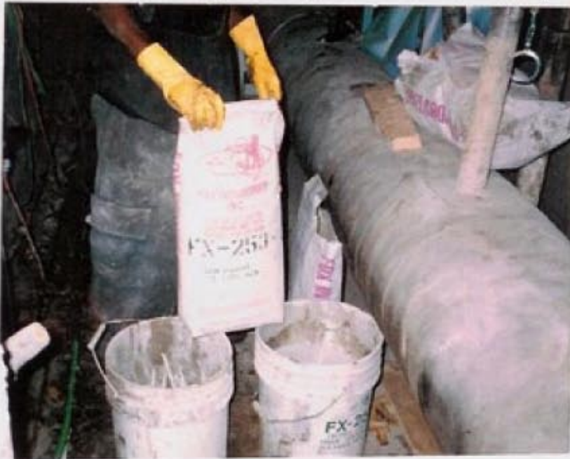
Small areas are patched with FX-792 LP Bonding Agent and FX-253 Trowel Grade Fiber Reinforced Polymer Mortar.
