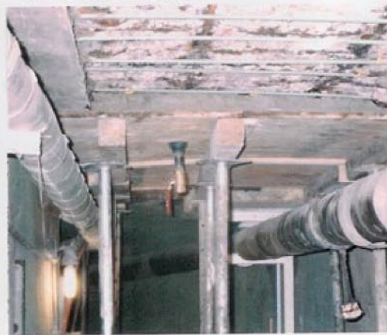
Large areas were repaired by placing temporary form work with pumping ports and pumping FX-228 Non-Shrink Non-Metallic Grout
