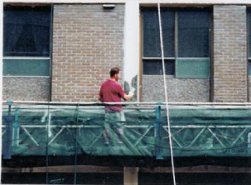
Columns and beams are repaired by removing deteriorated concrete. Exposed rebar is cleaned and protected with FX-408 Epoxy Zinc Rich Primer. The areas are patched with FX-752 Epoxy Bonding Agent and FX-253 Trowel Grade Fiber Reinforced Polymer Mortar. (over)
