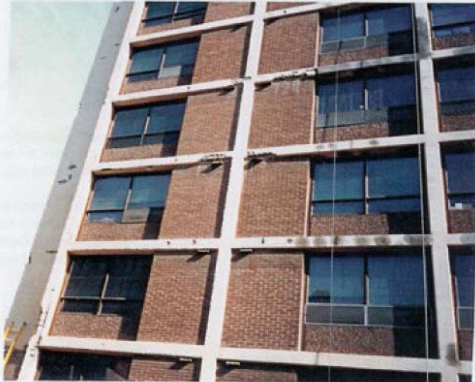
Seventeen (17) story high rise shown with work in progress. Moisture penetration caused rusting and expansion of rebar leading to rust stains, cracking and spalling of the concrete. Pieces of concrete fell from the building creating a safety hazard.
