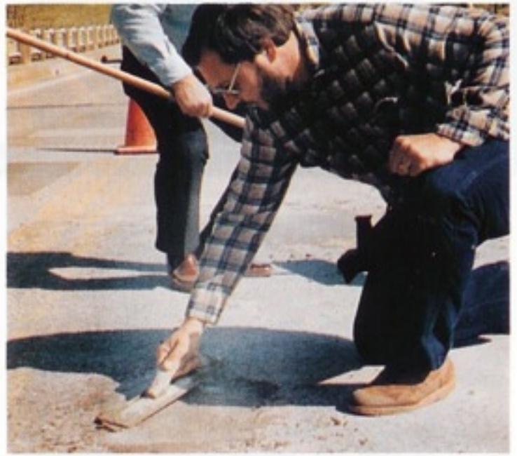
Mr. Jim Brown, Maintenance Contract Supervisor of Maryland D.O.T., assures that reinforcing steel is in proper position before FX-928 is placed.
