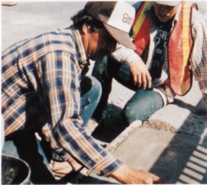
Mr. Ron Molesworth, Superintendent of Concrete General, Inc., repaired deteriorated sidewalk by skin patching with FX-928. He remarked that with the use of FX-928, the reduced amount of water was helpful when used in remote areas.
