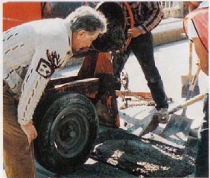
FX-928 is mixed and poured out into pothole. It is self-leveling with no gas bubbles.
